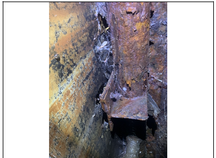
drain trough failed from corrosion
