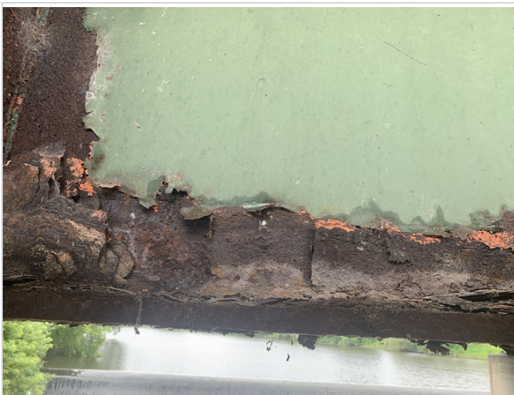
Section loss beam 1
