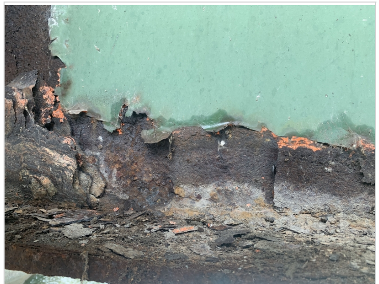
Heavy rust scale beam 1
