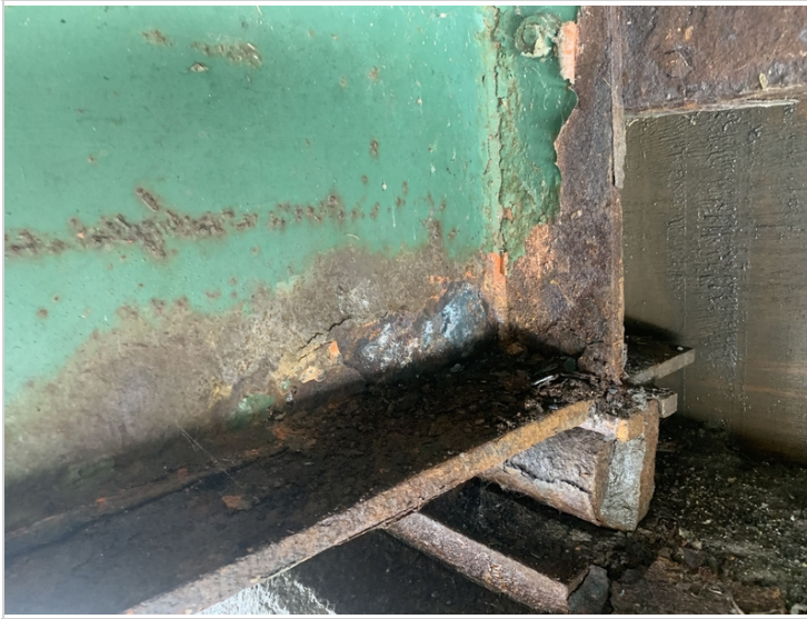
Section loss beam ends abutment 1
