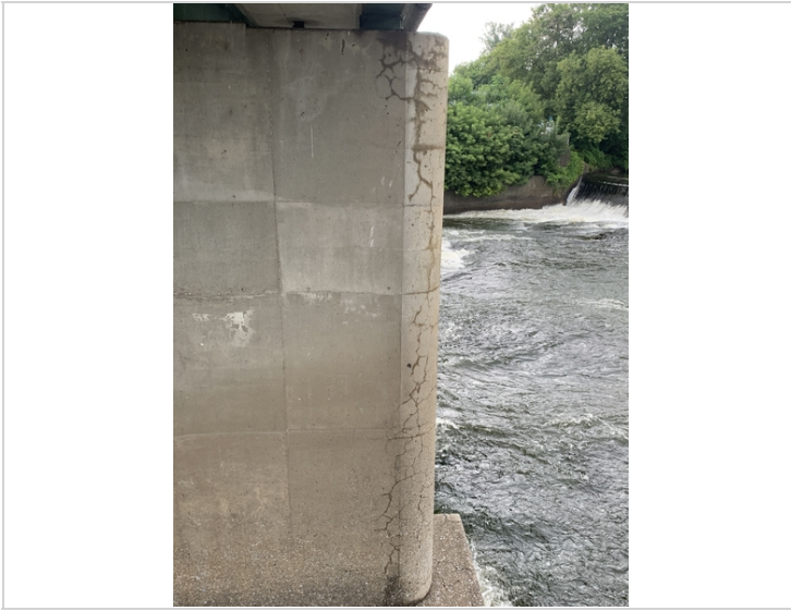
Upstream pier 2 nose cracking
