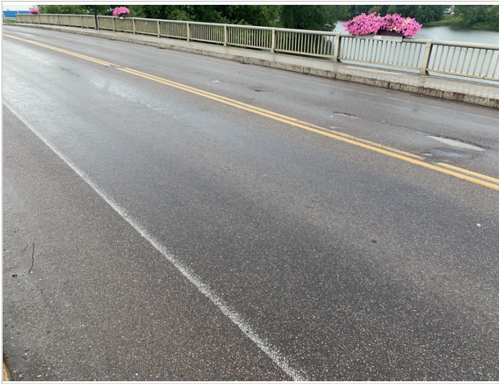
Potholes in wearing surface
