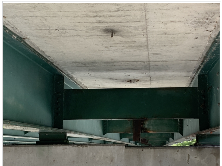
Saturation and minor spalling around deck weep tubes
