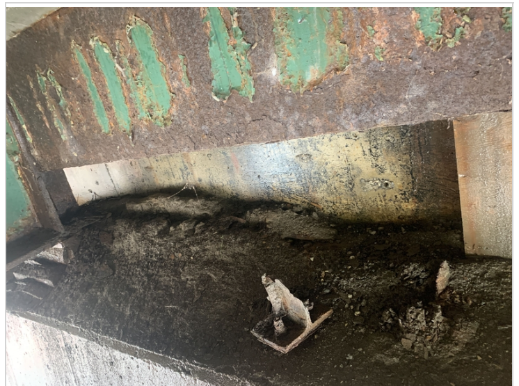
Debris on abutment 2 seat
