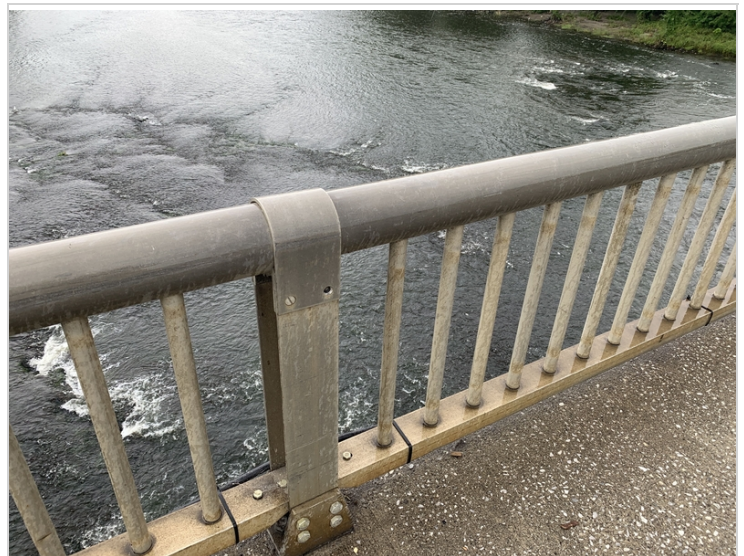
Missing bolt in the rail hoop
