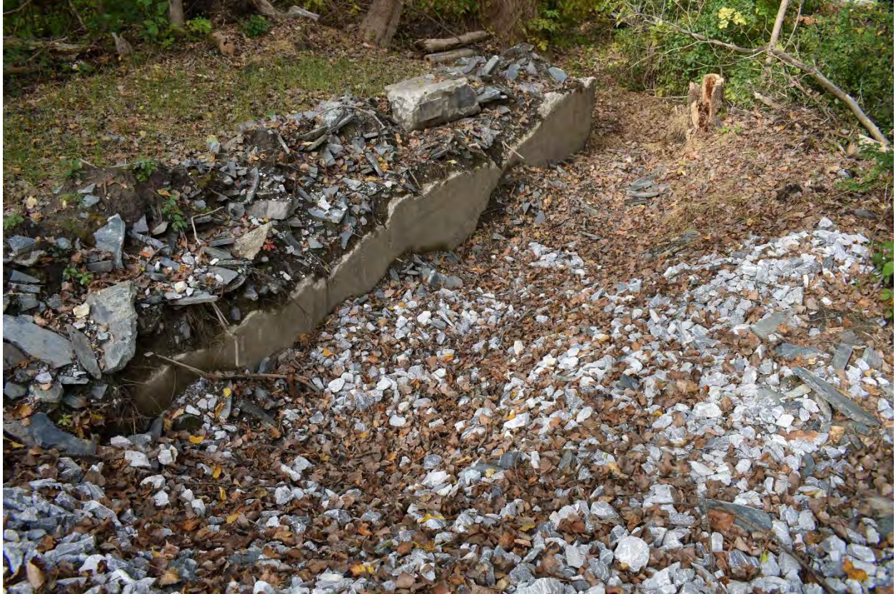
Figure 26. View northeast of the unidentified foundation located in the northeast quadrant of the proposed Swanton BF 036-1(16) Project in Swanton, Franklin County, Vermont. The foundation is located in ASA 6. Note the poor condition and the amount of marl scrap fill. The bridge is located to the left of and behind the photo.
