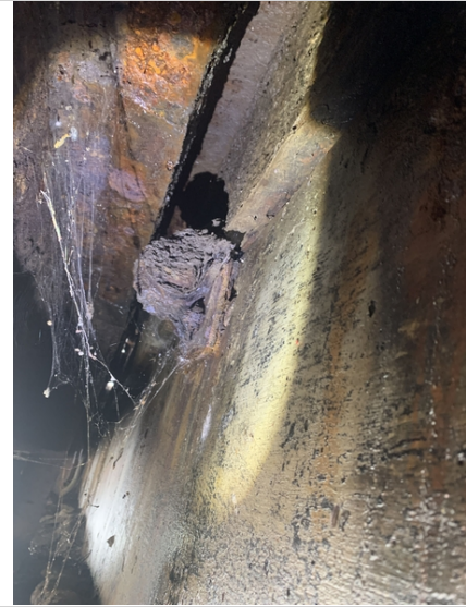
corroded bracket abutment 1 joint
